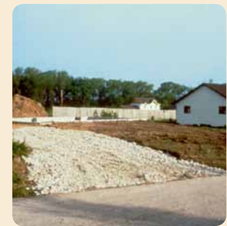
A gravel tracking pad is the designated unloading zone for trucks at this construction site. The gravel keeps dirt out of the street as trucks exit and enter.
