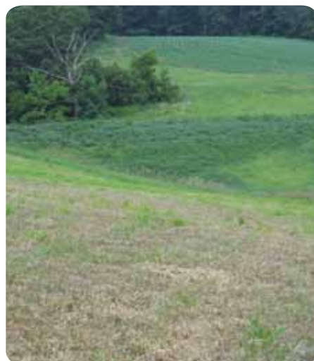
ABOVE: At the Barkheim Farm near Stockton, Minnesota, this catchment basin was cleaned out and repaired with Stockton-Rollingstone-Minnesota City Watershed District funds. It captures moving water and soil where a field meets a ravine, to prevent flooding and erosion.
